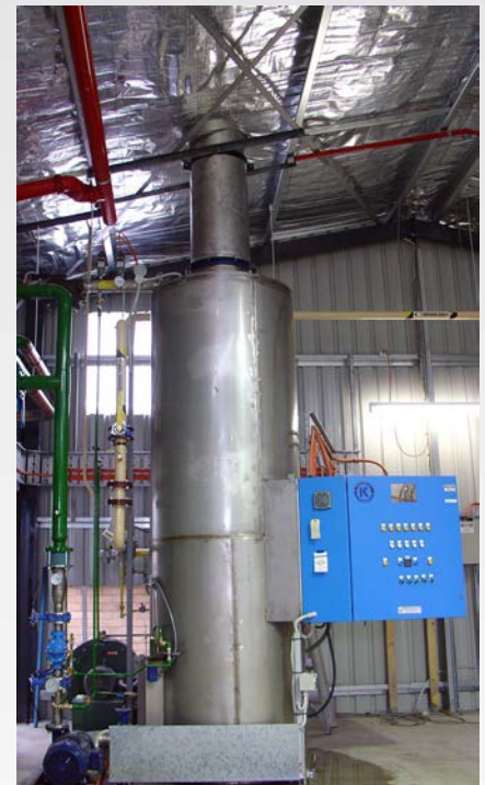
Direct Contact Water Heater (DCWH)
